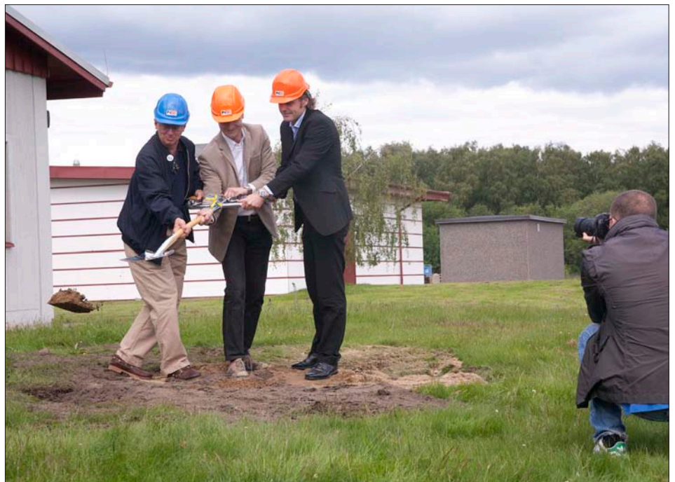
The first turf for the expansion is cut by Municipal Commissioner Lars Ahlqvist, the construction company's CEO Tobias Persson and Nolato MediTech's MD Johan Iveberg.
