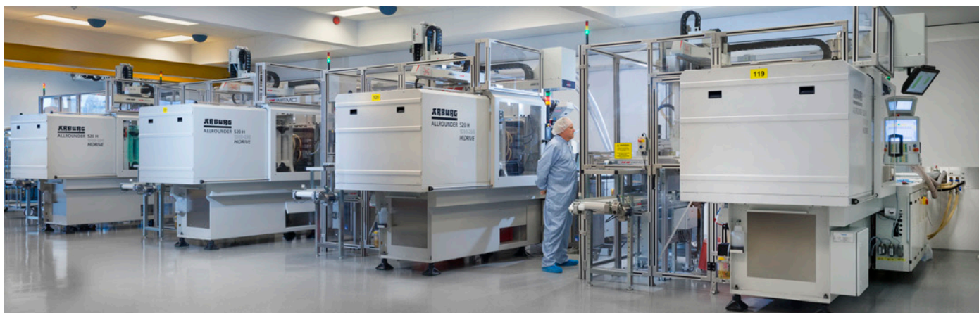
The new clean room has an efficient system for supplying injection mould machines.
