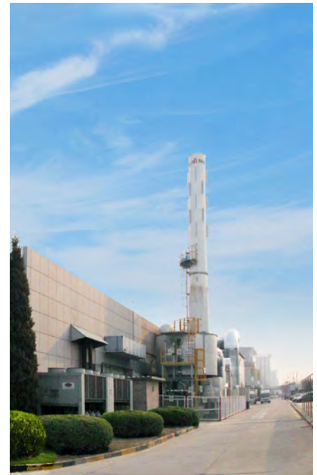
A new air emission abatement equipment at Nolato's painting facility in Beijing was installed in 2014.
